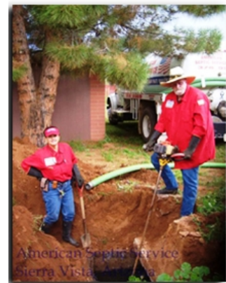
Photo courtesy of American Septic Services.
